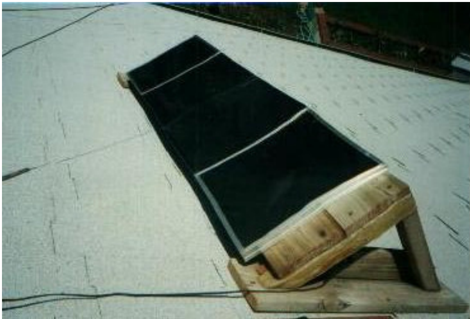
Solar panel on the roof
